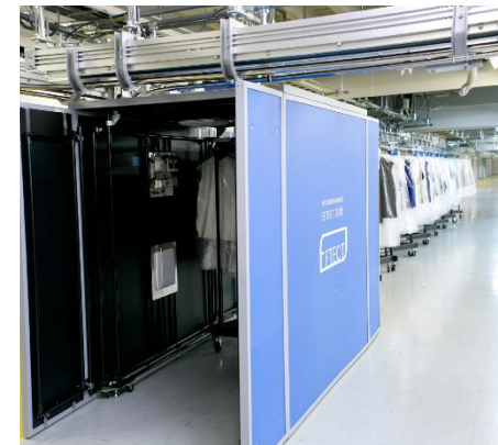
Installation of tunnel gates capable of reading a batch of RFID tags at once
